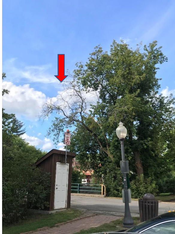
Figure 11: A priority 1 prune, deadwood overhanging a street (red arrow).
